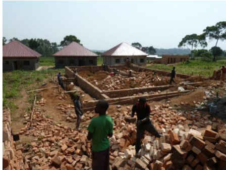
The foundation for our teammates' house-ours will be next to it and identical
